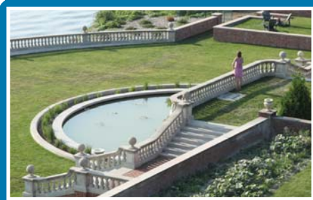
2012 saw structural repairs completed on the Lily Pool as part of the ongoing Formal Gardens Restoration Project.
